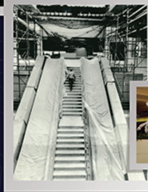
New Center Escalators
